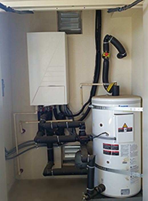
Typical electric HVAC and hot water heater closet at Mutual Housing Spring Lake.
